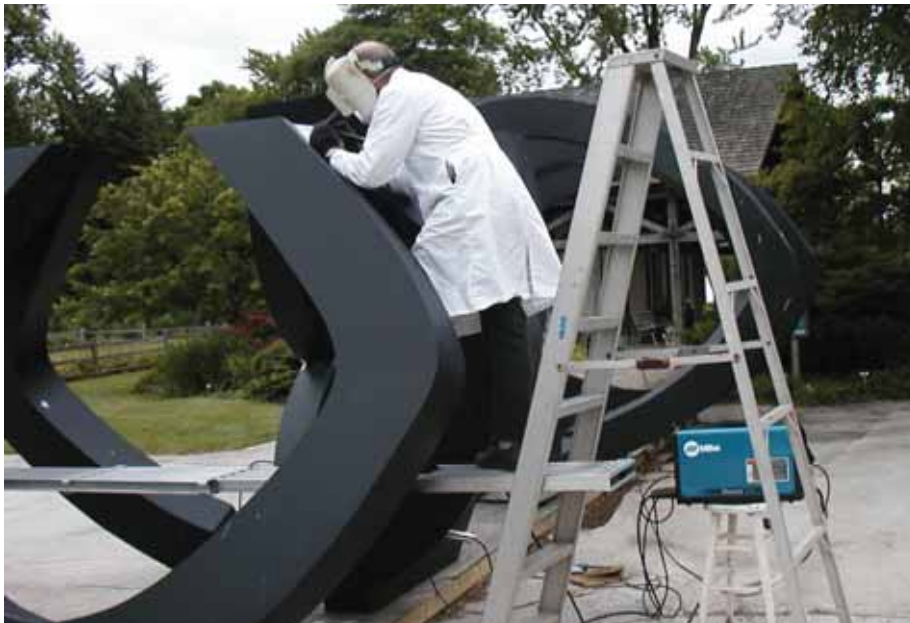
The Dynasty 200’s Auto-Line capabilities enabled Joe Canfield to make this field repair simply by changing from the 460 volt, three-phase plug used in the shop to a 230 volt, single-phase plug.
